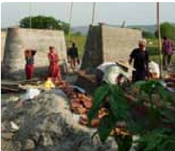
▲ Locals constructing new bridge at Meghauri, Chitwan to improve their accessibility during the flooding season.
