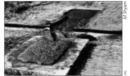
Figure 3: Discharge pits of the modified plants: the top pit has an unaltered outlet channel – the lower pit has a channel which has been made wider
