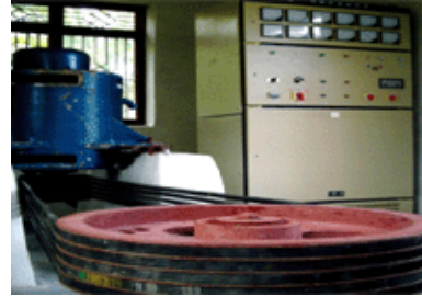
40 kW Imported Turbine
