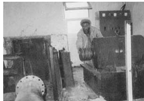
Generator at Pari micro-hydro plant, Gilgit
