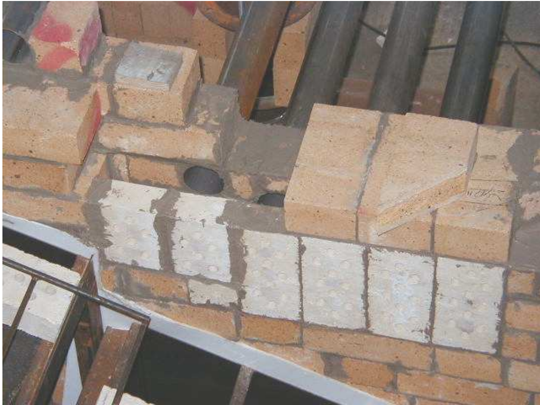
Figure 3.9: Building side air plenum
