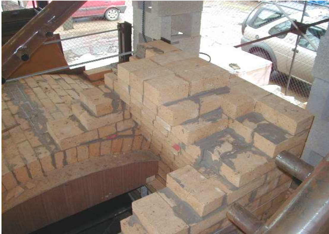
Figure 3.13: Cross connector built on top of primary chamber roof-arch - showing corbelled wall under construction and secondary-air tubes (view from ash end)
