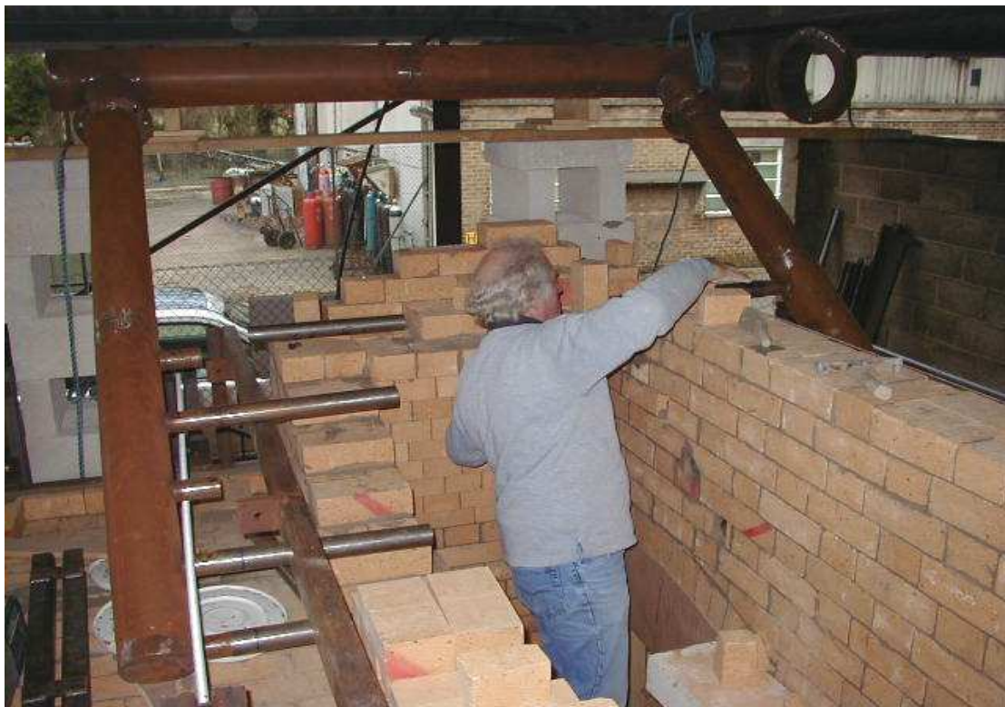
Figure 3.14: Building up the vertical walls of the cross chamber from the corbelled end
