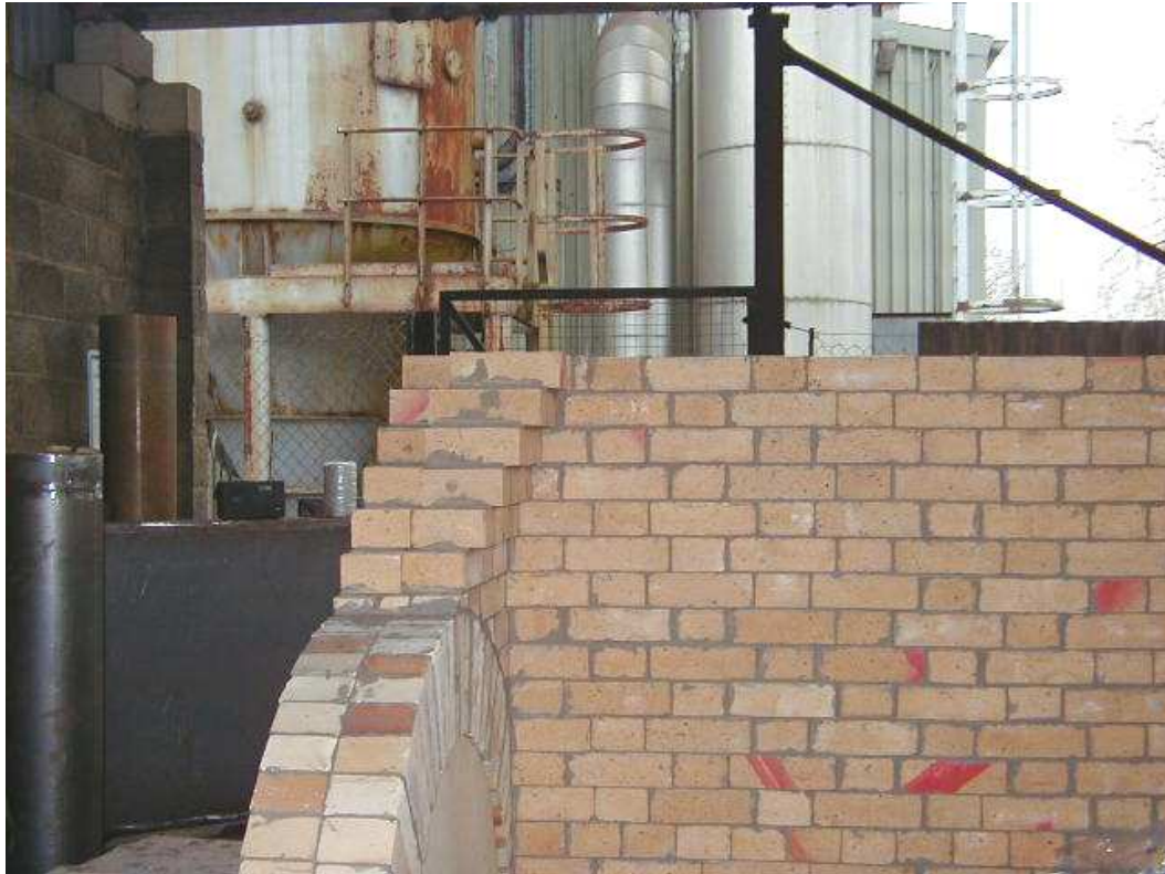
Figure 3.8: Corbelled wall above access arch on Ash End wall of the primary chamber
