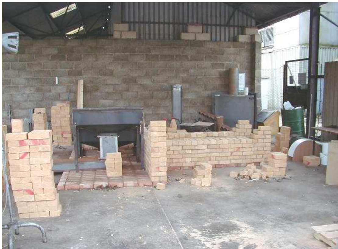
Figure 3.4: Building primary chamber right hand position (Note: Plenum/grate shown is the prototype design and differs from current design)
