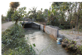
Reinforced concrete wall lining was introduced as a measure to avoid flood intrusion into communities in Sonaha, Geruwa Municipality.
