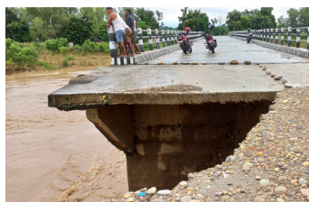
Damaged approach section of a bridge in Phanta by the flood in September 2022.
