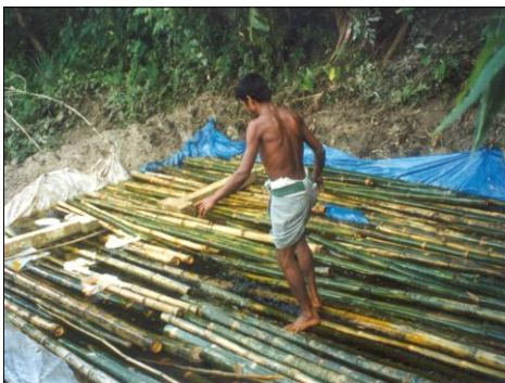
Figure 4: Curing bamboo trees for building flood resistant houses Faridpur, Bangladesh. Photo: Practical Action Bangladesh.
