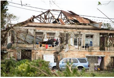
Photo: destruction of houses after Cyclone Idai, Mozambique, March 2019 by Denis Onyodi/IFRC-DRK-Climate Centre.
