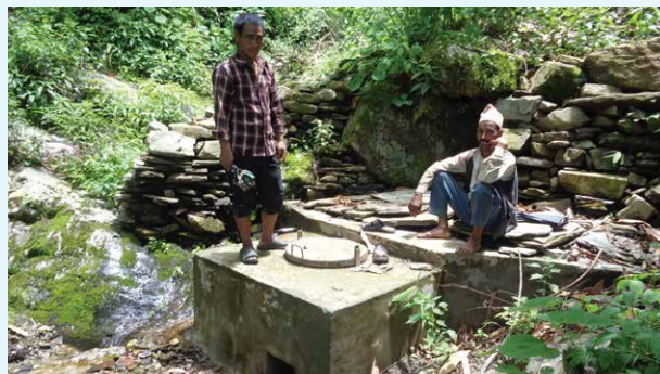
PHOTO 3: WATER INTAKE OF GHARIHOLA DRINKING WATER PROJECT
