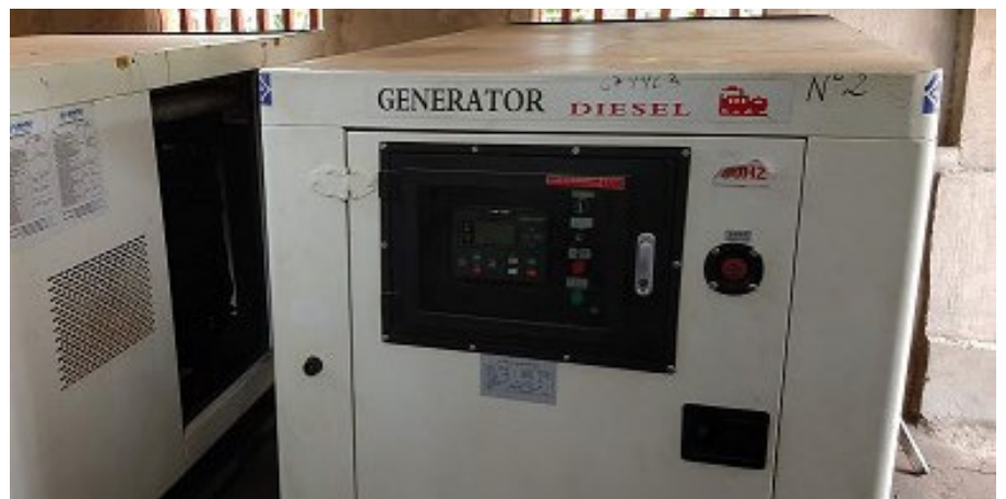
Photo 2 Nyabiheke camp generators
